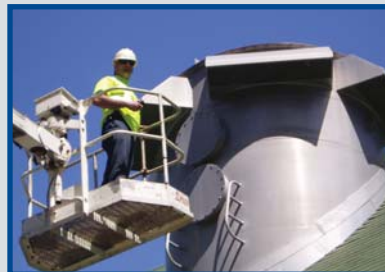
Ken Podlaski performing annual maintenance on one of the District's five air stripping facilities.
